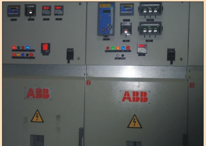
Sub Station, Srinagar
